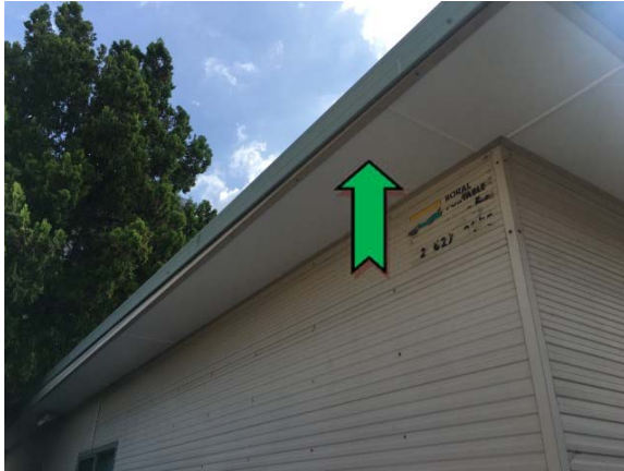
Photo 1. Exterior, throughout, eaves – non asbestos-containing fibre cement sheeting and suspected lead-containing white upper paint systems.
