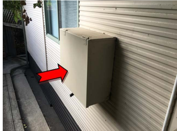
Photo 2. Exterior, north elevation – suspected asbestos-containing bituminous backing board.
