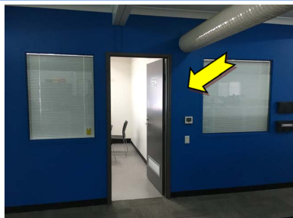
Photo 12. Interior, throughout, southern wall – suspected lead-containing dark blue upper paint systems.
