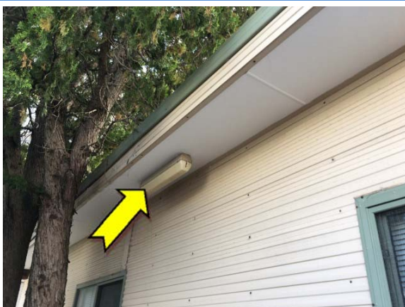
Photo 11. Exterior, throughout, single tubed fluorescent light fitting – suspected PCB-containing capacitor.
