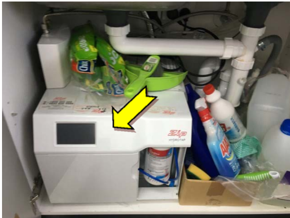
Photo 9. Interior, kitchen, under sink hot water heater – suspected SMF internal insulation material.
