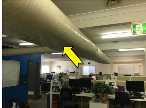
Photo 8. Interior, throughout, ductwork – suspected SMF internal insulation material.
