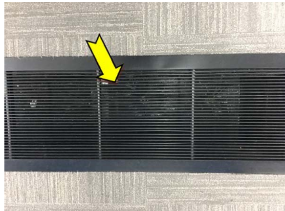
Photo 10. Interior, throughout, subfloor, air conditioning duct work – suspected SMF internal insulation material.
