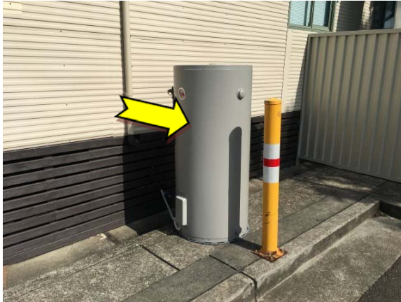
Photo 7. Exterior, north-east elevation, hot water heater – suspected SMF internal insulation material.
