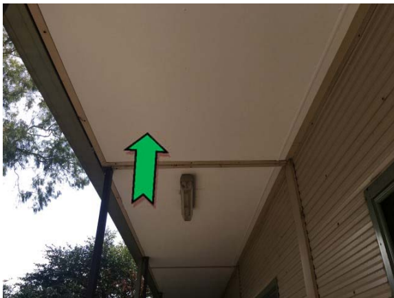
Photo 3. Exterior, north elevation, awning – assumed non asbestos-containing fibre cement sheeting and suspected lead-containing white upper paint systems.
