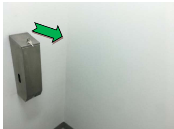
Photo 6. Interior, female toilets, south elevation, wall – assumed non asbestos-containing fibre cement sheeting.
